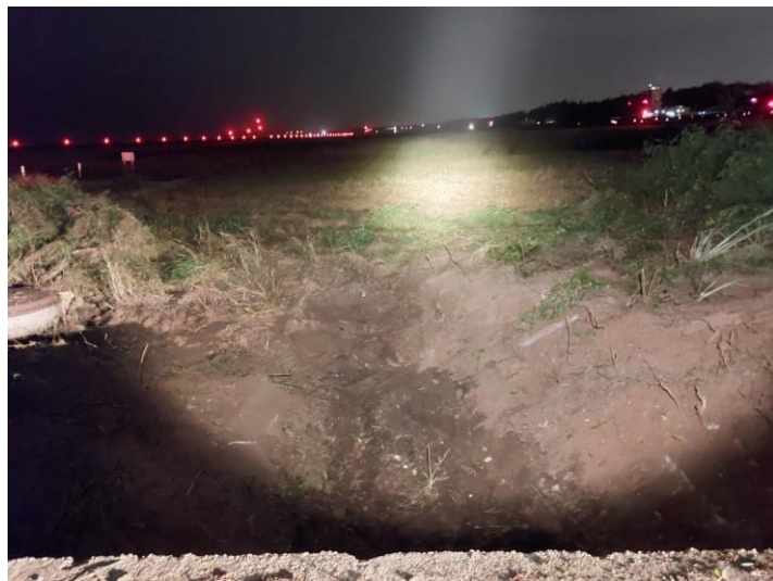
24 跑道頭凹坑填補 (改善前)圖-7
